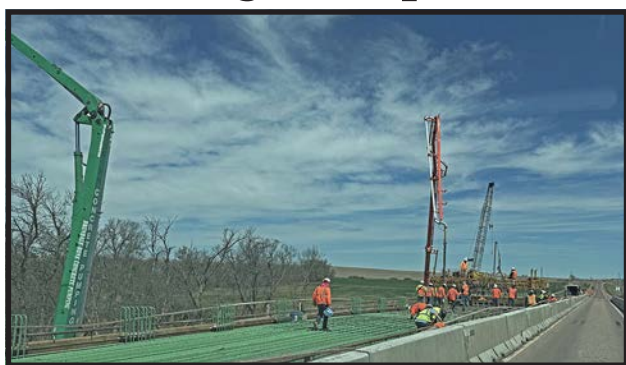
The bridge construction north of Hoxie on Hwy 23 was finally pouring the concrete last week. It won't be long before it will be open to traffic. (Sentinel Staff photo)
